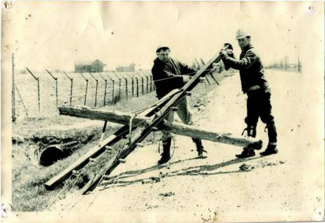
A newspaper article from the Citizen in May 1966 shows the devastation of a sleet and wind storm that went through the area. Shown here are two employees of the Hay Municipal Telephone System, Bill Wagner and Lloyd Denomme removing downed telephone lines from Highway 81 in front of Bell Aerospace, southeast of Grand Bend. Three or four miles of lines were destroyed in that particular area, while losses in other sections were as bad or worse.
