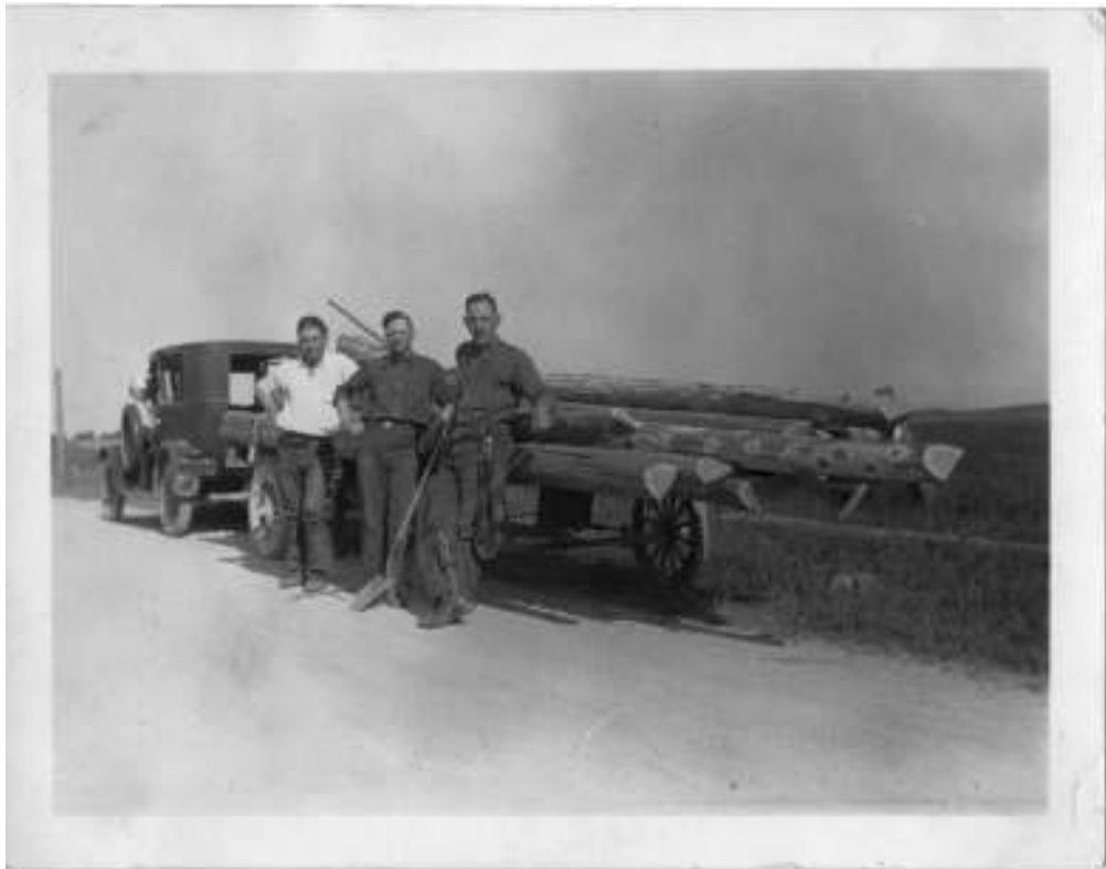
Taking a break from setting telephone poles. From the left (both photos): Leonard Wagner, Edgar Wuerth and Harry G. Hess.
