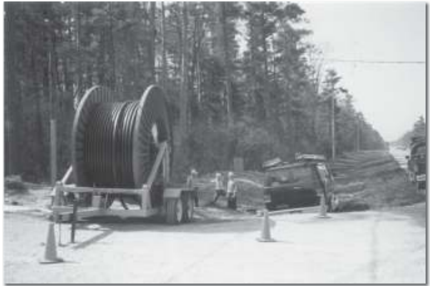
New subdivisions requiring more lines means upsizing of existing facilities. 612 meters of 900 pair cable pulled all at once. From left, Rick Fisher, Marty Merner and Steve Meidinger, May 1992 at Merrywoods subdivision.
