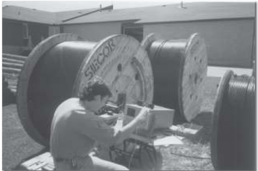
Kevin Mulvale of Fiber Optics Canada was brought in to assist with the fibre installation. In this picture Kevin is testing each fibre strand before they are put into the ground.
