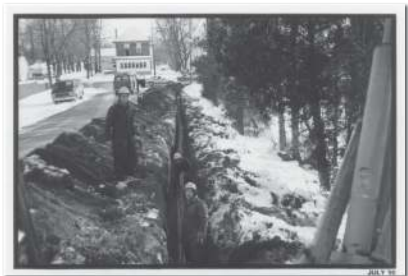
Rebuilding of Oak St., concrete-encased duct structure. Working in the trench are Hay staff Ken Clarke in front and Erich Freiter behind. On the bank is Terry Zehr, front and Keith Semple.
