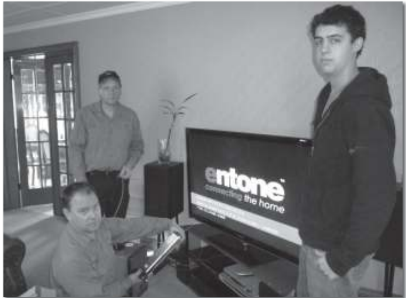
From the left standing is Joe Hendriks, kneeling, Rob Rau, and Coop Student Jason Masse install a set-top box required for IP Digital TV service.
