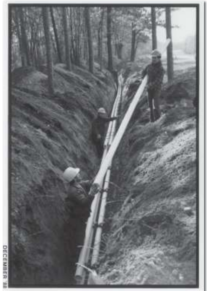
G.M Gest Construction contracted to install concrete encased duct structure. Photo taken at Severn Park adjacent to Huron Woods looking south to the Klondyke remote office.
