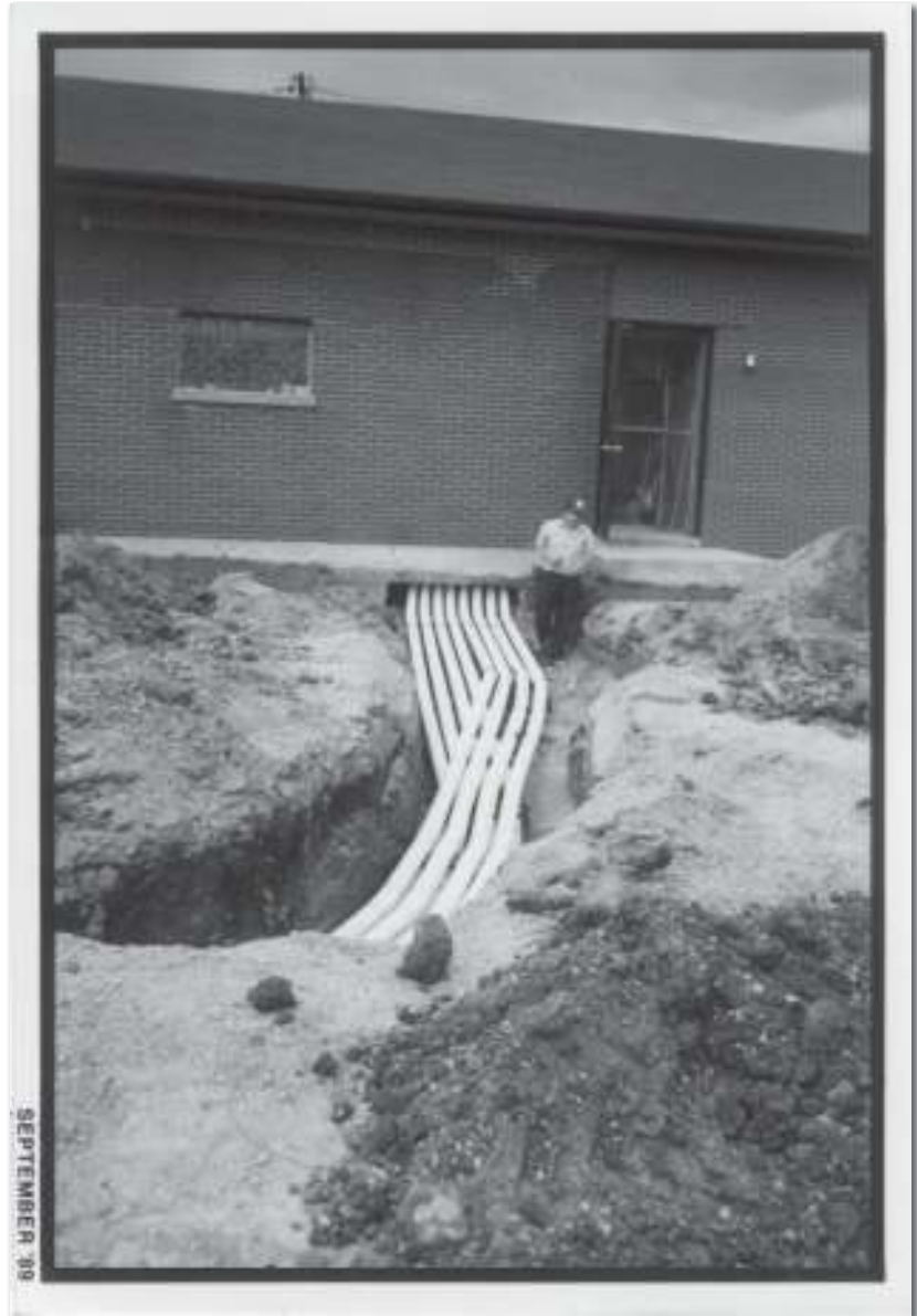
Ken Clarke stands by the Grand Bend "CO" as multiple ducts are installed.
