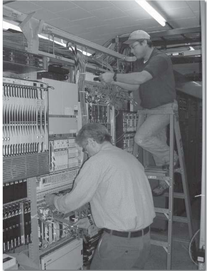
Upgrades continue with the installation of the new CS1500 softswitch in the Dashwood "CO" in 2008. Keith Semple standing and Kevin Gingerich on the ladder.
