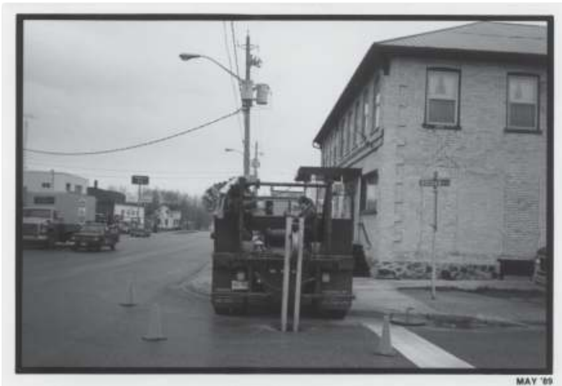
In front of the Dominion Hotel in Zurich, Marty Merner preps the winch preparing to pull cable. .....
