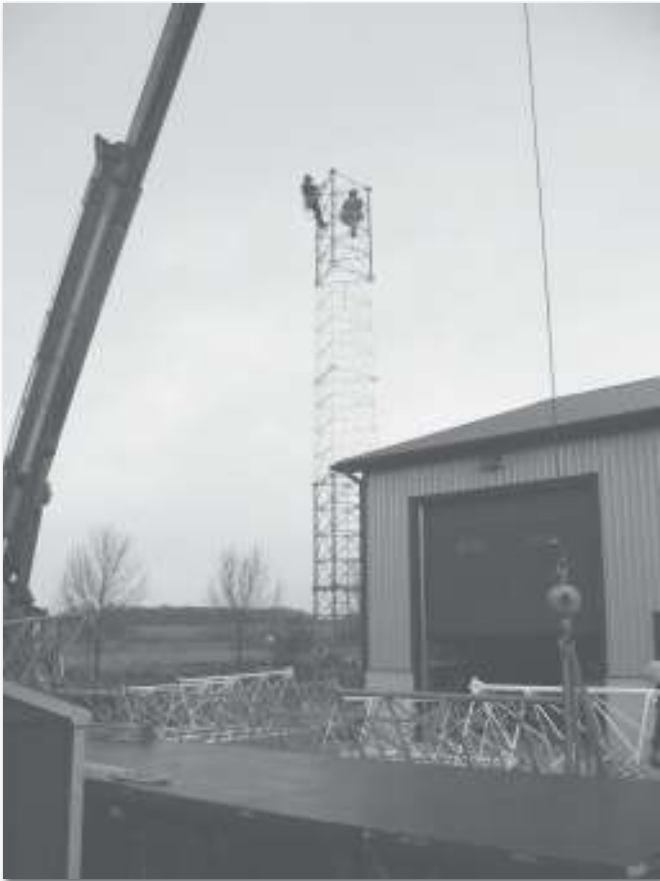
Advanced Tower workers erect a wireless tower at the Zurich Business office that will provide cellular service in Hay's territory.
