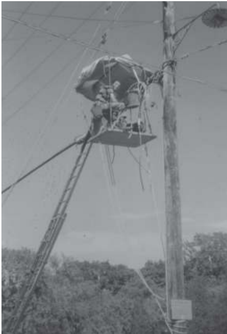
An aerial tent. This unknown Hay employee hauls up all his tools and even a heater if necessary to work on a cable splice. The sides of the tent can also be dropped down if needed. The photo was taken in Grand Bend.
