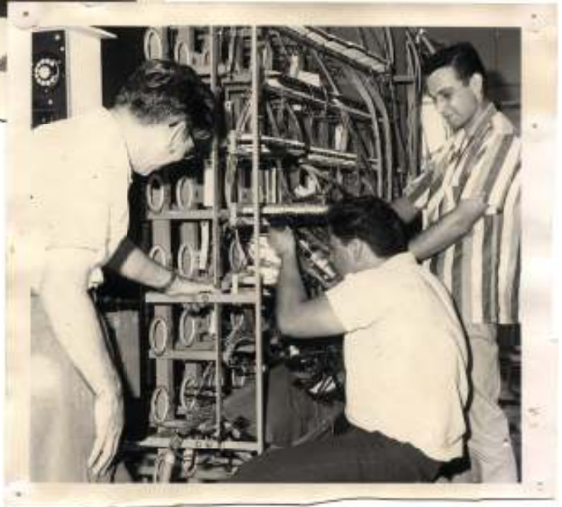
A November 1966 newspaper article accompanying this picture stated "Delicate Operation – The installation of dial equipment in the Dashwood exchange of the Hay Municipal System is a touchy operation, and requires the highest quality of skilled men to do the work. In this photo supervisor Jim Orr, left, of Northern Electric, is watching the work being done by Art Martin, centre, another employee of the same company. At the right is Bill Wagner, an employee of the Hay System. The dial exchange is to be completely ready for the cut-over by the middle of October." .....
