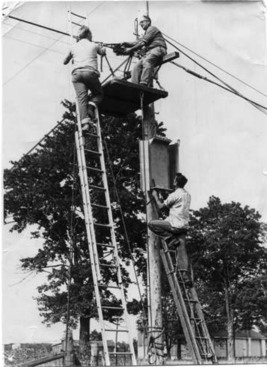
Constructing and splicing an aerial terminal, contract splicer Jack Keller of Seaforth (on the elevated work platform) is assisted by Hay employee Bill Ingram while Ivan Meidinger preps a "Ready Access Cabinet". .....
