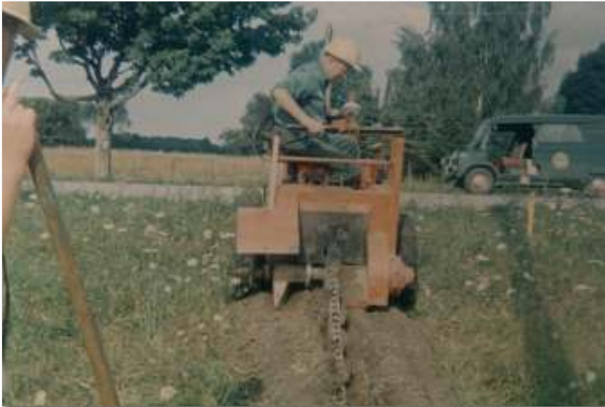
Taken in the early 60's Jack Keller is at the controls of his trenching machine installing new underground cable. In the background a nice look at the Bedford van that was used during that time period. .....
