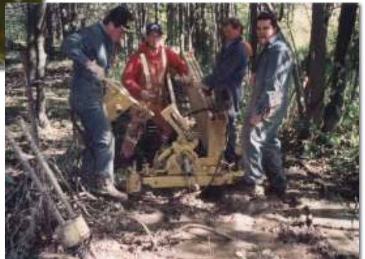
Subjected to adverse conditions. In 1993, Weber Contracting is directional drilling conduit under Mud Creek along Hwy 83 through Hay Swamp. Shown here are from the left: Erich Freiter, Darrell Konings (Weber Contracting), Rick Fisher and Marty Merner.
